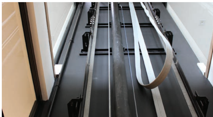
CUSTOM PAINTED MECHANICAL
